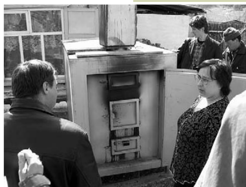
E. Potorchina, director of Solnyshko Kindergarten demonstrates a new boiler unit installed under the project
