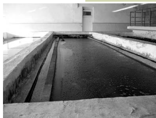
Before an ultraviolet disinfection system was installed at the water inlet of Ussuri Rehabilitation Center, chlorine had to be used at the water treatment station, which significantly lowered the properties of the water supplied to ten thousand local residents and guests
