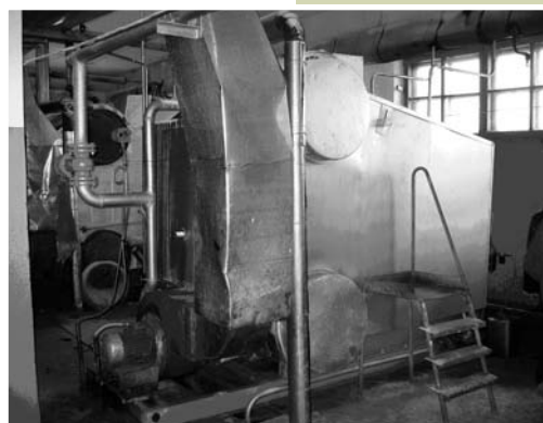
The boiler plant in Plastun settlement is being converted from the use of diesel fuel, for which a lion's share of the municipal budget is spent and which severely pollutes the air, to the use of wood waste
