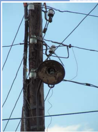
Several dozen of such 1970s street lamps were replaced with new modern ones in the settlements of Babino Rural Municipality
